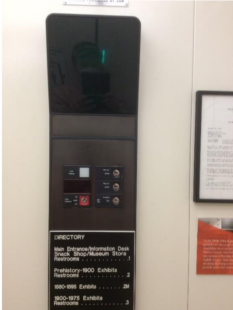
Car 4 control panel
